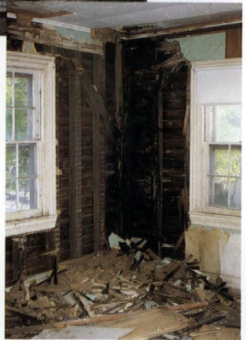
This series shows why it is impossible to guess the extent of structural damage without opening up the structure: (Top) The appearance of the interior wall prior to tear-out. (Middle) The damage revealed after removing aluminum siding. (Bottom) A roof leak has completely rotted and washed away the 4x6 oak corner post. This is why change orders exist.
