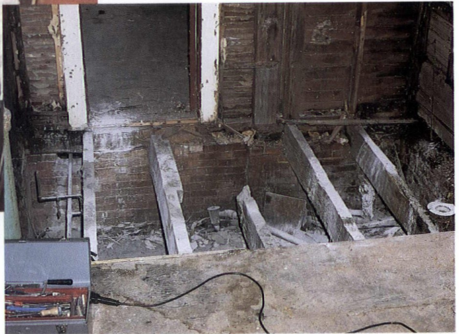
In the photo above, a much-abused bathroom awaits renovation. Like a dentist removing decay from a tooth, the rot is slowly peeled away until the only thing left is the floor joists (coated with lime to kill the smell). Because hidden problems can sometimes reach this extent, most contractors will bid a job of this sort as time-and-materials.
