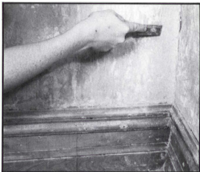
If the underlying plaster is sound, a chisel can be used to scrape off unwanted texture finish.
