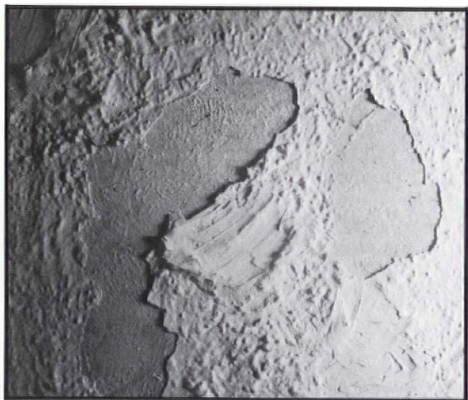
Failing texture finish that will have to be scraped and perhaps steamed.
