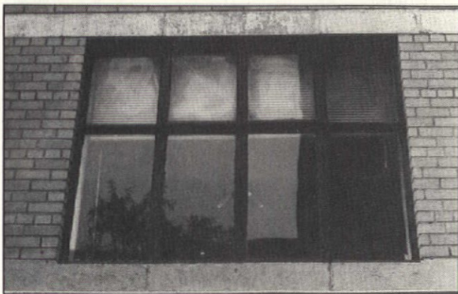
Metal windows in the city: metal-clad Kalamien windows on an apartment building.
