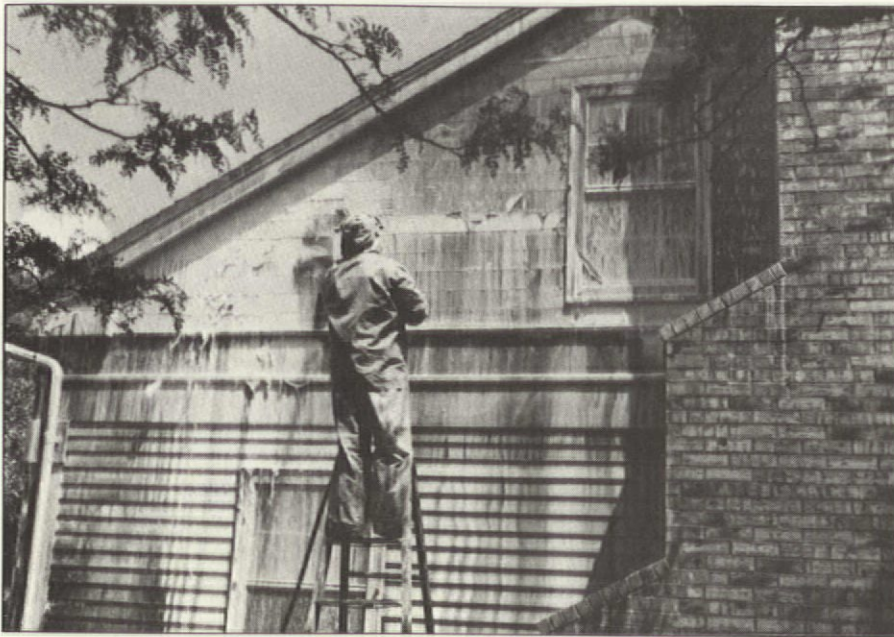
Here's the wholesale approach in progress. A workman rinses effluent from clapboards that had been coated with chemical stripper.
