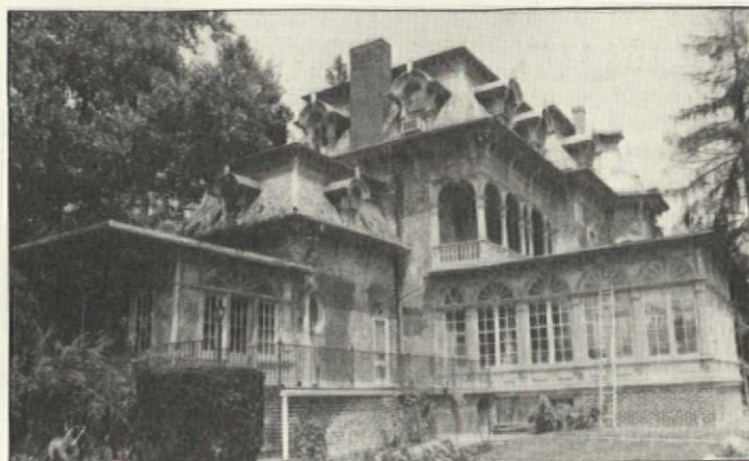
The owner intended to repaint anyway, but look what stripping revealed: patches, bad pointing repairs, and wood trim.
