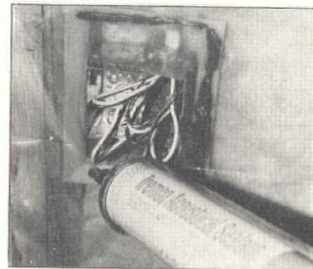
Plastic vapor barrier is sealed around boxes and edges with non-hardening Tremco Sealant.
