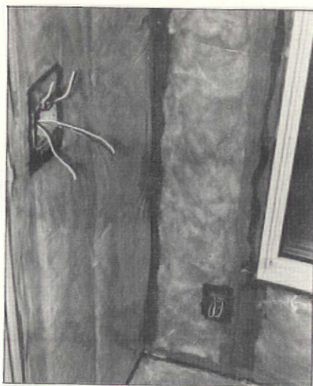
Air/vapor barrier film and boxes are shown sealed into place over insulation.
