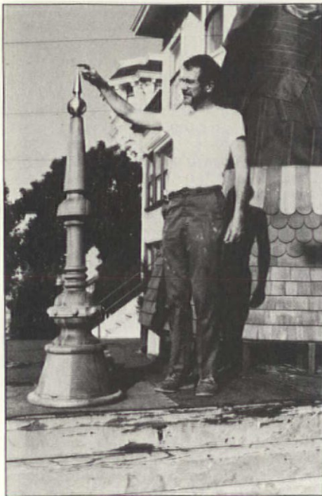
The soaring redwood finial has a 14-lb., turned stainless steel tip that acts as integral flashing as well as a pigeon dissuader. The tip is a lightning rod, too; the steel is welded to a threaded pipe which goes through the wood finial, then is screwed from inside to anchor it. A grounding cable runs to earth.
