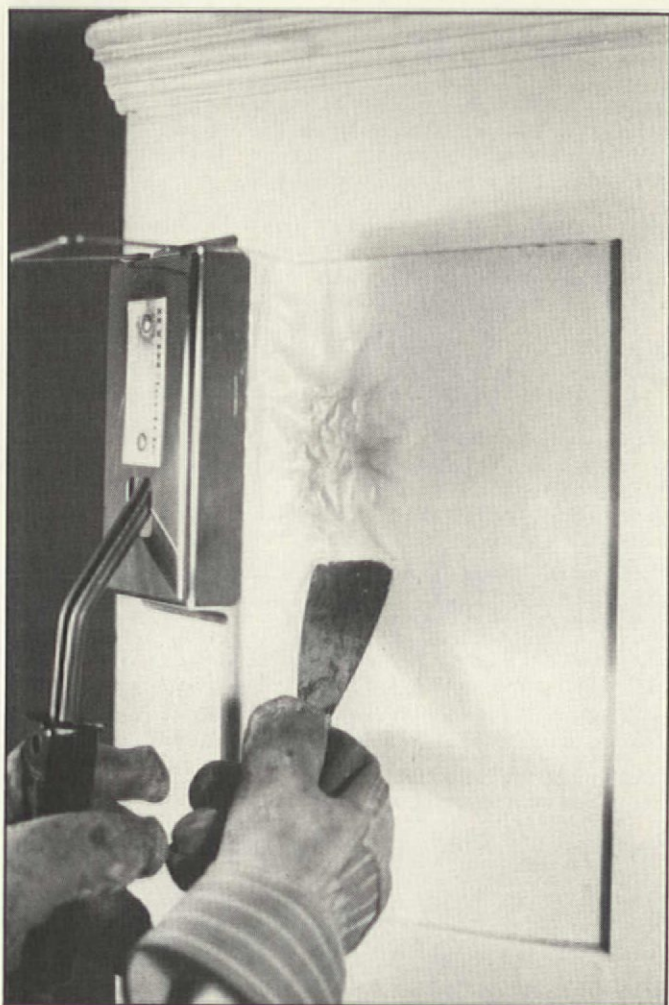
A Hyde electric heat plate is being used to loosen paint from the surface, forming a large bubble behind the paint.
