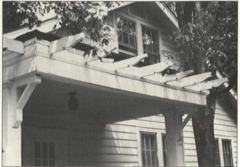
Sneaky rot: Previously repaired rafter ends were visibly rotten. After the gutters were removed, it became clear the whole roof was rotten, interior framing and all.
