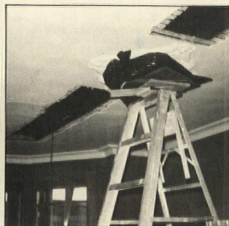
A drooping plaster medallion, shown propped in place with padding. Plaster of paris was poured over the top to re-key it.
