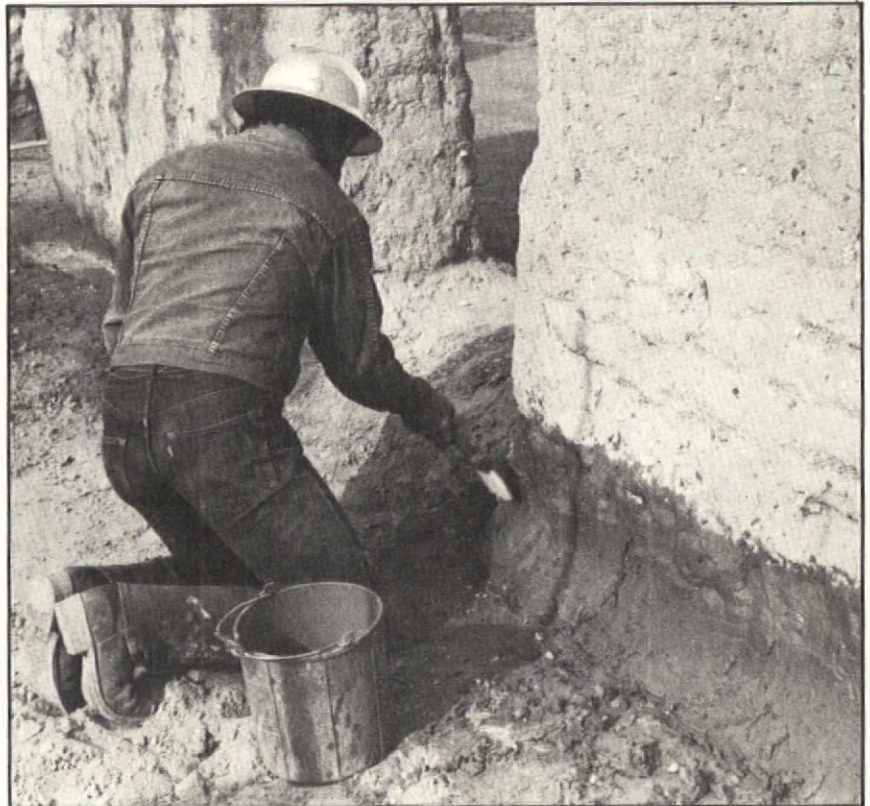
Adobe plaster is being applied to the base of this eroded wall.
