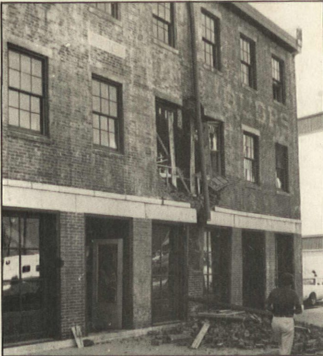
THE PILE OF BRICKS that fell from the front of this building undergoing renovation was an ominous sign that the gods who protect old buildings were not pleased with what was going on inside. Just a few hours later . . .
