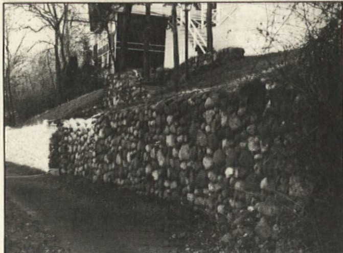
BEFORE: This handsome fieldstone wall blended neatly into its surroundings. And then the painters came along...
