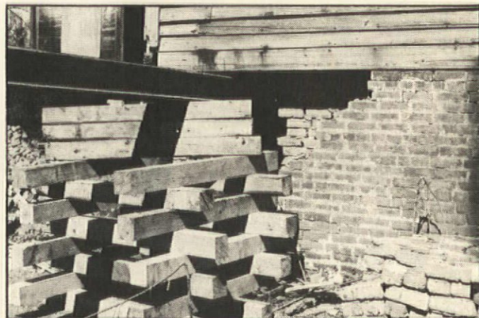
Another view of the Greiss house just before its relocation. Here the steel beams are being cribbed up as the foundation is removed.
