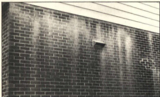
Excessive chalking of the paint from the clapboards caused this streaking on bricks.
