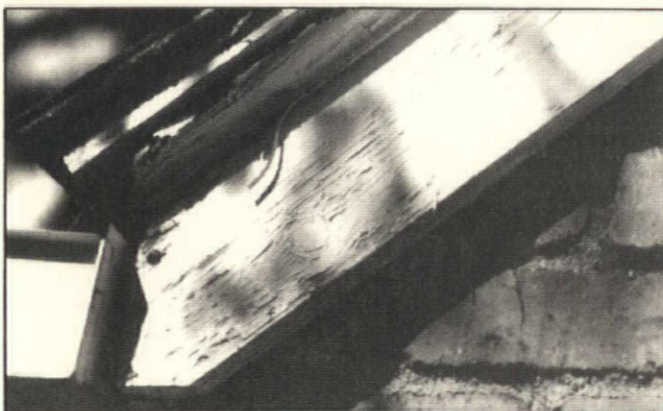
Another exciting paint-failure photo: Not merely inter-coat peeling, but cracking and peeling down to bare wood, due to moisture.
