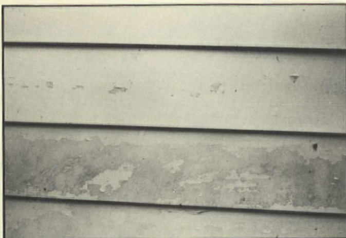
The factory finish on this aluminum siding had faded and peeled years before. The owner had been maintaining a regular painting schedule.
