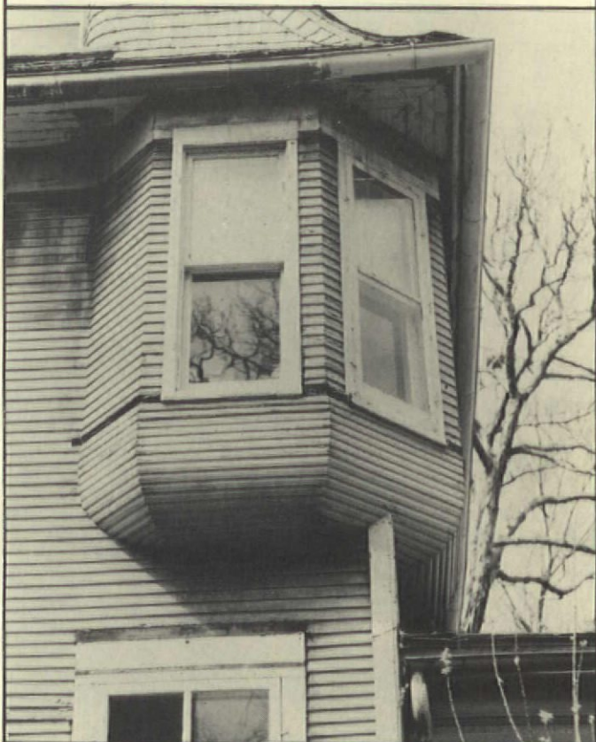
With the replacement siding off, the original proportion of the beaded wood clapboards is apparent. A trim board at sill level was discarded during siding installation.
