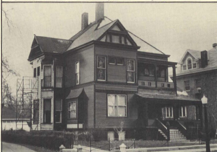
Here the siding is being removed. On the facade, deteriorated and missing boards were replaced, painting has begun, and the porches are being restored.
