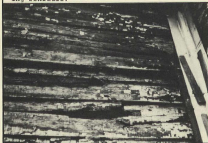
This deterioration was caused by the aluminum siding. Studs were rotting, and interior plaster was damaged.
