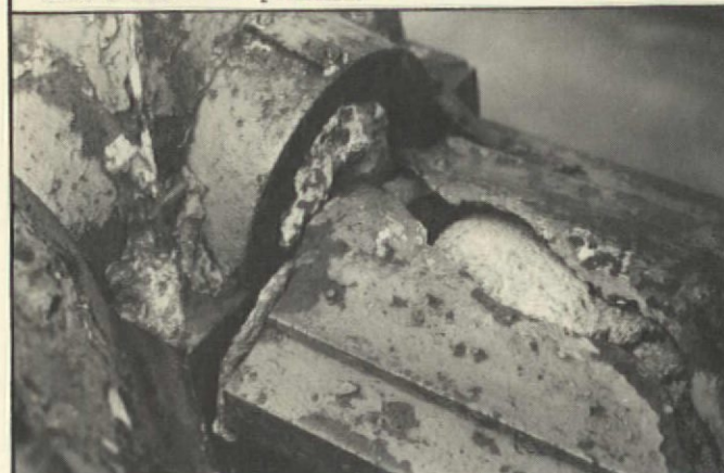
Example of exfoliated iron--expanded by rust--due to filling with concrete.
