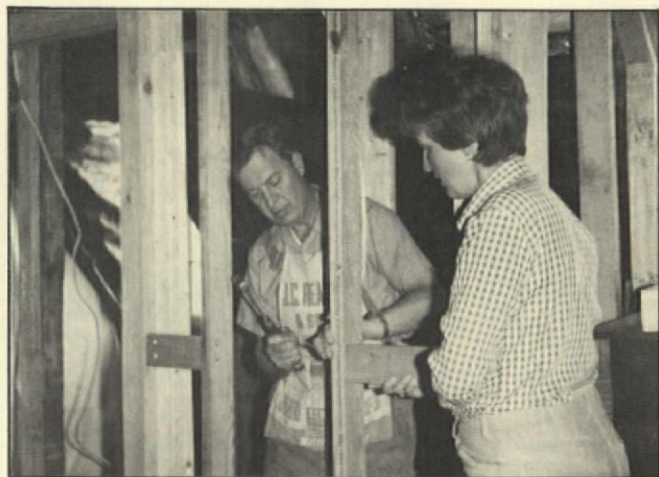
Dean and Gail completing rough-in of upstairs bathroom in the master bedroom.
