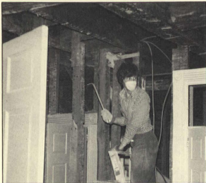
Gail is removing the last of the lath and plaster in the corner of the dining room.
