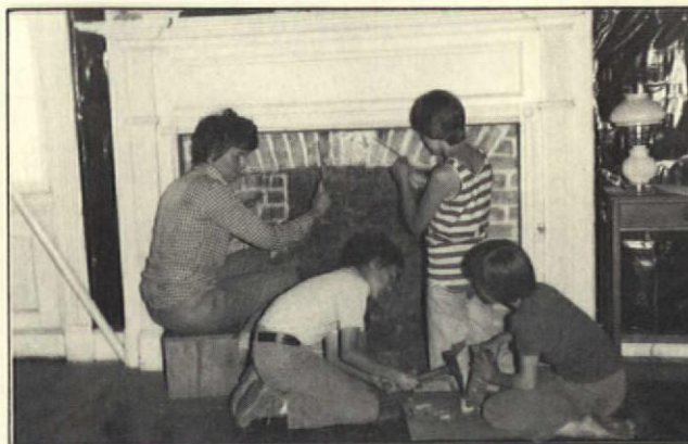
Laura, John, Nancy and Gail tuckpointing fireplace in dining room. John is cleaning original bricks before replacing.
