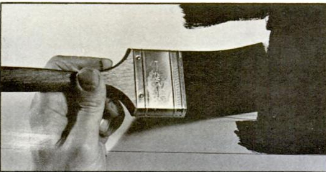
2. Limits of stencil band are measured onto wall, and lines established with a chalkline. Background color is then painted into band. We used a flat oil-based paint.
