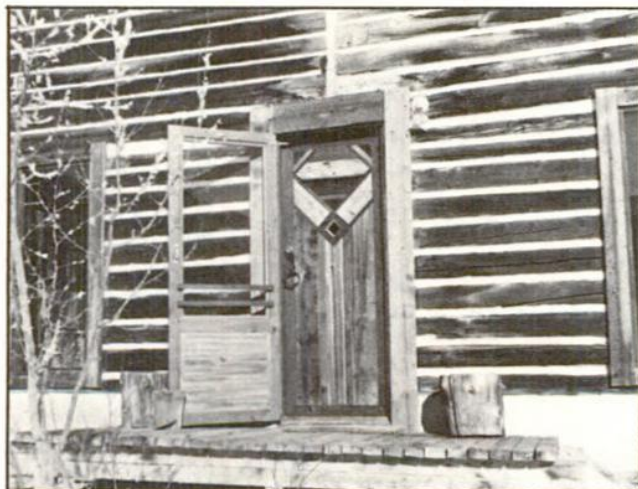
The smooth chinking can be seen in this view of the front of the house. Peter made the front door pattern out of varied shades of wood. Almost all the wood used in the restoration is native spruce and pine felled nearby.
