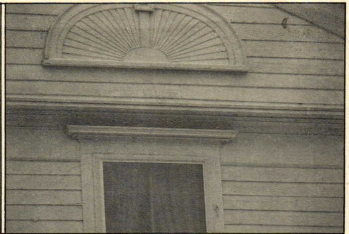
dow and created the cap on the window cornice to match the original woodwork (shown on the window at the right).
