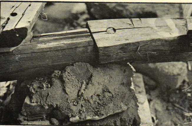
Lap joint in one of the original locust girders—resting on rebuilt footing.
