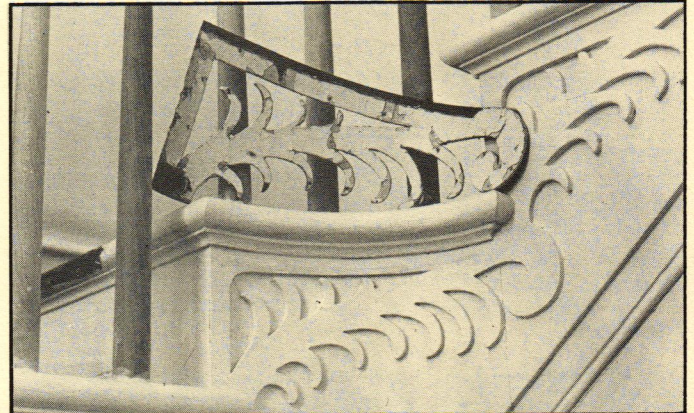
Original decorative brackets on curve in stairway were made of leather to accommodate the bend. (One of the originals is shown propped on the stair.) Missing pieces were duplicated by laminating 1/8" poplar.
