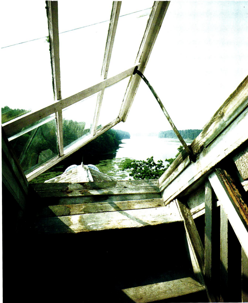
At Georgian-period Hamilton House in South Berwick, Maine, a skylight-roof vent in the attic proves that this practical idea is nothing new.
