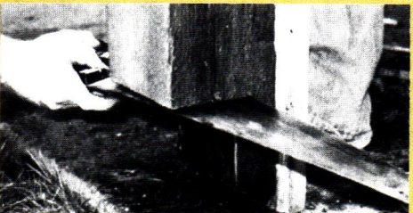
10" rotted bottoms of these load-bearing columns...
