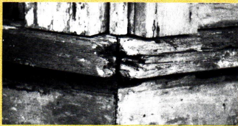
This rotted - and irreplaceable - woodwork...
