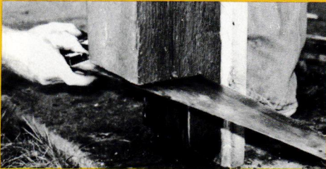
10" rotted bottoms of these load-bearing columns...
