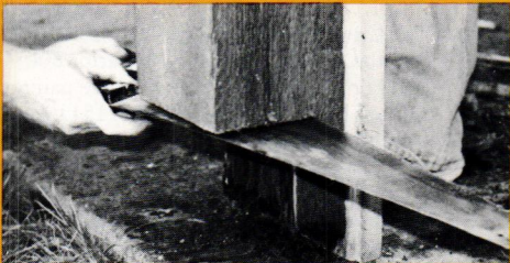
10" rotted bottoms of these load-bearing columns...
