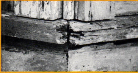
This rotted – and irreplaceable – woodwork...
