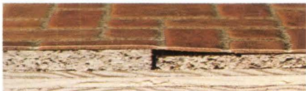
Tredway continuously adjusts to seasonal subfloor movement.
