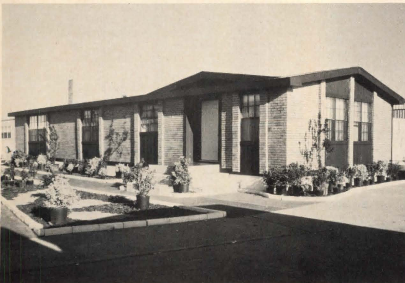
Simulated brick siding (above) is produced by applying an "auto-mark" tape or "quick-set" template over a mortar base and then troweling over a texturing compound. Brick/Master, Lake Forest, IL. Circle 262 on reader service card
