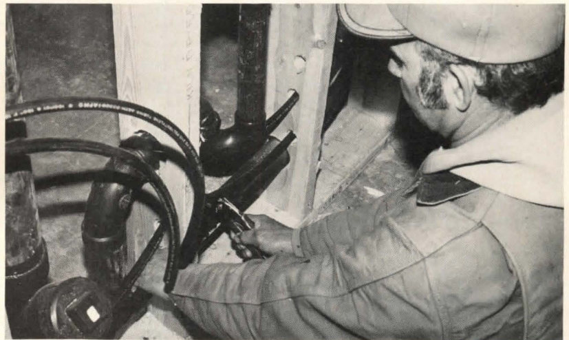
Installation is cheaper, quicker and easier with polybutylene piping than with copper, says builder Millard Scudder of Indiana. He says he has used new pipe in 60 homes.
