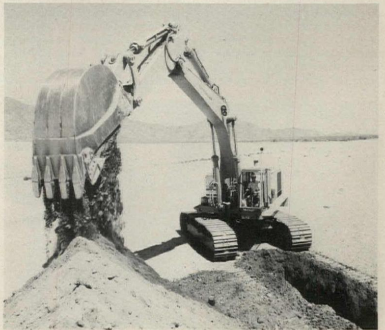
Hydraulic excavator has a sealed track-type tractor undercarriage. The "245," with standard 10'6" stick, has a maximum reach of 41'10" and a maximum digging depth of 28'. Five bucket sizes are available. Caterpillar, Peoria, Ill. CIRCLE 262 ON READER SERVICE CARD
