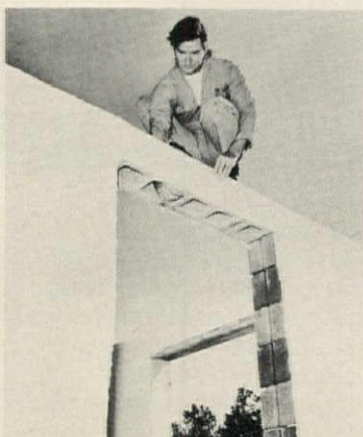
Surface bonding cement secures concrete blocks without the use of mortar. Blocks are laid in a regular pattern, aligned, and then the vertical surface troweled evenly with an \frac{1}{8} " thickness of surface bonding cement. The white cement matrix, which is embedded with fiberglass strands for strength, has good holding power and is highly resistant to weather and moisture. Stucco-like finish of the cement requires no further coatings but can be painted with latex. Bonsal, Lilesville, N.C. CIRCLE 223 ON READER SERVICE CARD
