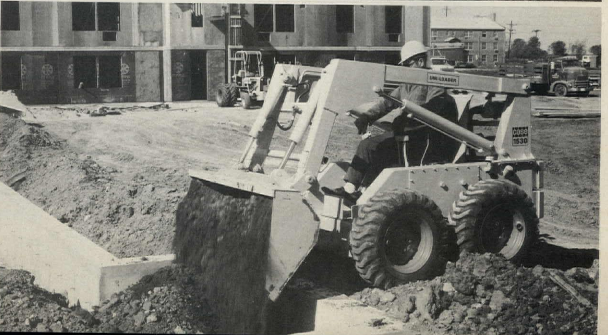
Versatile loader is only 5' wide, gets between trees or into tight areas, turns 360° in its own 6½' length, and lifts 1500 lbs. up to 9½' high. Besides lifting with the adjustable pallet fork or dumping with the bucket (one of 17) shown, it is also a dozer, drills post holes, shears trees, plows snow, digs trenches and sweeps streets. Case.
