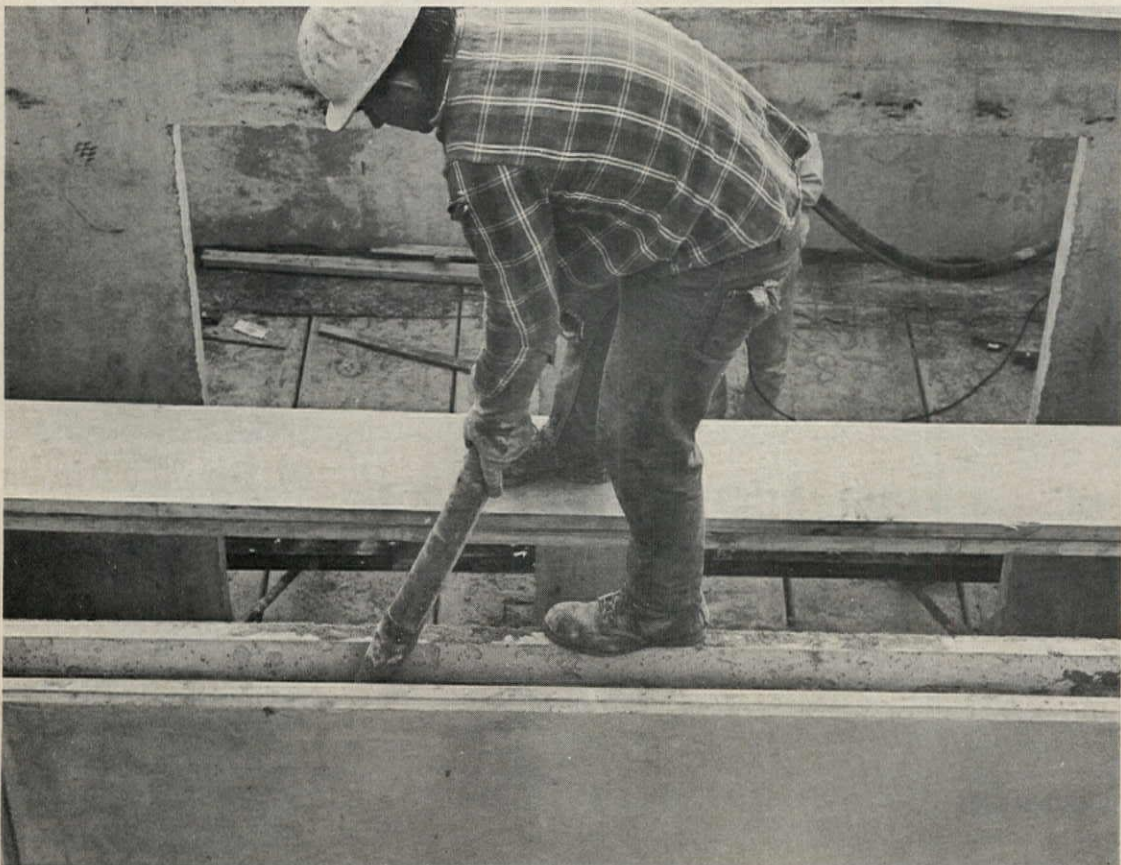
Grout is pumped into wall-panel voids to form continuous key between floors and walls. Hollow core pumice block floors have concrete topping over them. For second housing project, builder used prestressed lightweight floor slabs.
