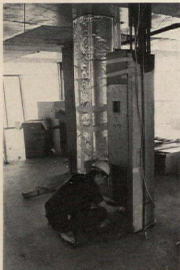
Maintenance is performed through upper and lower registers on unit.
