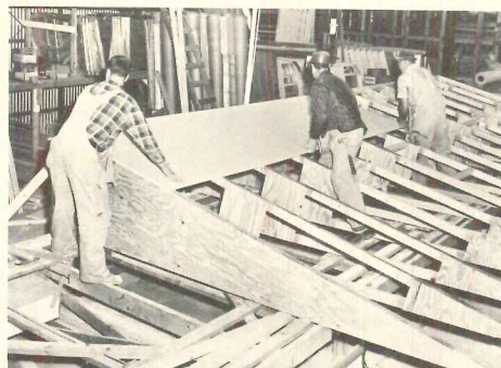
ROOF TRUSS SYSTEM has ceiling panels nailed to joists before assembly is installed.
