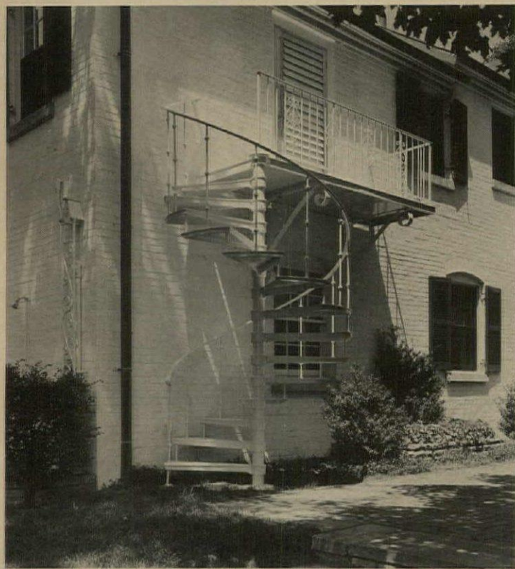
Spiral stairs come in many stock sizes, plus custom packages like the one shown, for indoor or outdoor use. Standard 4' diameter fits small areas. Treads install in right- or lefthand spiral. Logan, Louisville, Ky. Circle 230 on Reader Service card
