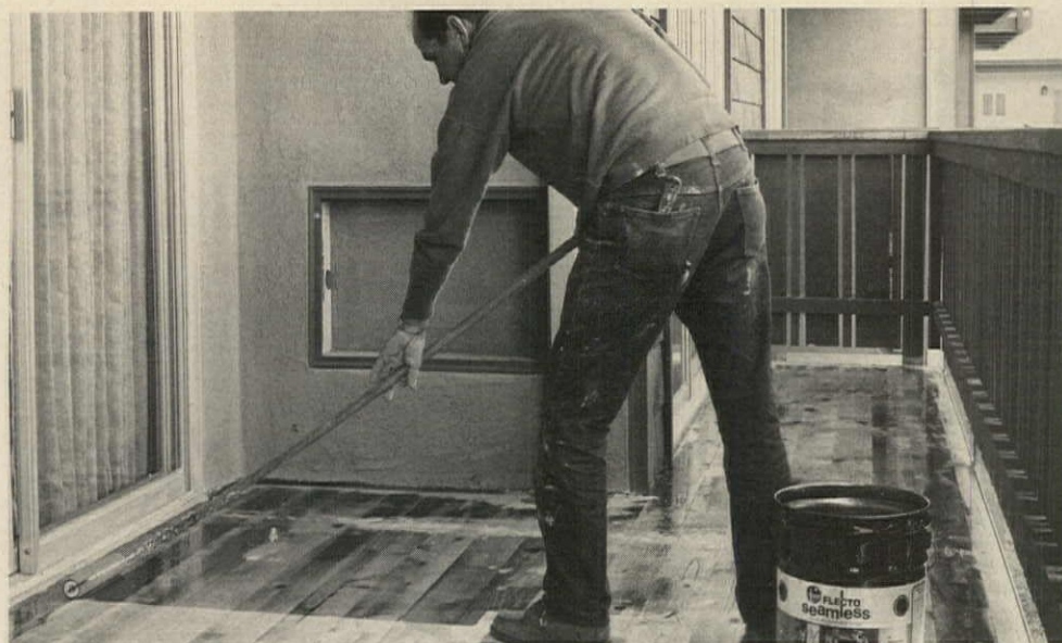
SEALING wood decking with clear laminating plastic is step one in applying seamless flooring.
