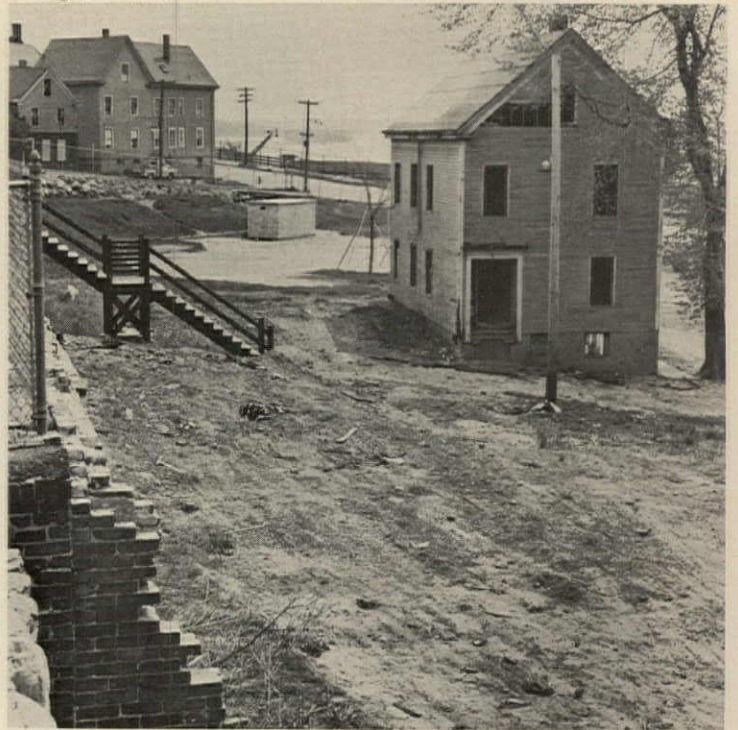
CLEARED LAND shows site's steep slope and original retaining walls, which were kept whenever possible. House at right was torn down.
