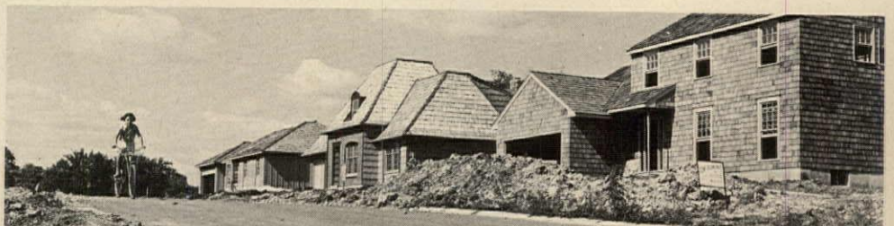
UNFINISHED HOUSES. like these being built by Tom Redmond, were scattered throughout Kansas City during summer-long plumber's strike. Redmond was opening new subdivision with units priced at $25,000.
