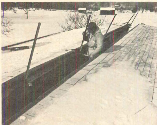
1. JACKS are evenly spaced under roof section of a Capital Industries house shipped with a 2-in-12 pitch.
