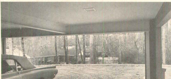
CLEAR-SPAN CARPORT (6) is supported by two steel I-beams, which carpenters installed. Installed cost: $160.
