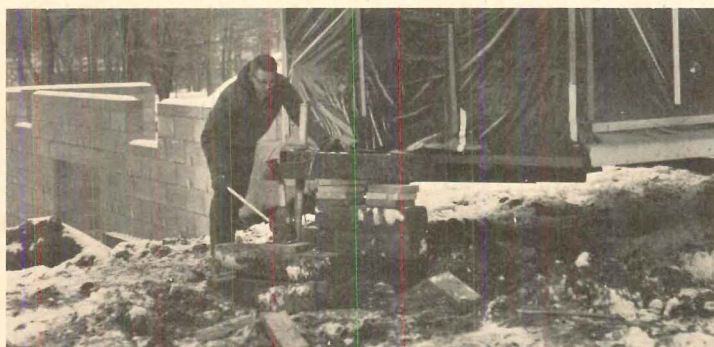
3. JACKS and cribs are set under house section's steel perimeter beams, and lifting starts. Under ideal site conditions, total lift is only 4½".
