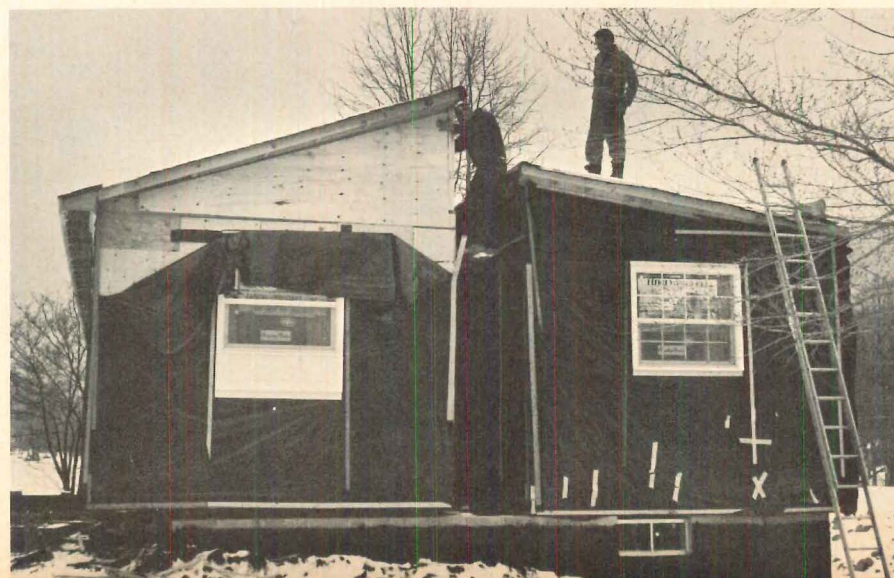
4. GABLE-END PANEL is inserted and nailed. House sections remain 2' apart for roof work.
