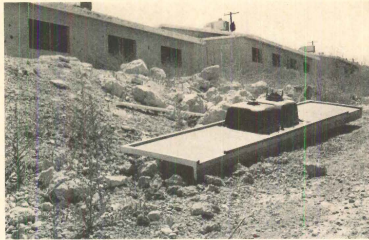
INCREDIBLE VANDALISM , such as this sink ripped from vacant 52 units of Hilltop Apartments, depresses market. Apartment vacancies top 17%.
