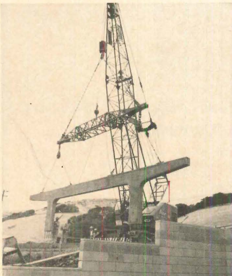
HEAVY CRANE made precasting of tees uneconomical, forced builder to cast them in place.
