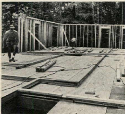
SIMPLE SYSTEM starts with plates on sub-floor. Studs are toenailed and tilted up.
