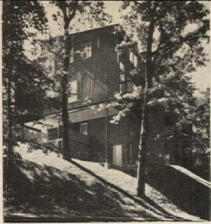
DOWNHILL MODEL. seen here from back of the site, has partly excavated basement.
