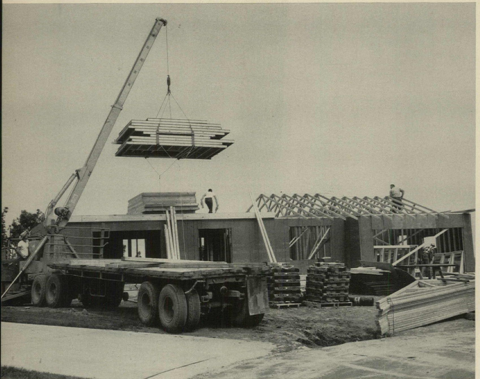
BOOM TRUCK , which cost Pemtom $13,000, hoists panels to deck of two-story house, which has one-story wing including garage at right.
