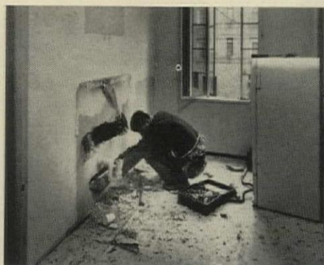
4. OLD KITCHEN is ripped out at 8 a.m. on first day of remodeling. Old refrigerator is kept in operation right up to replacement. Workman immediately runs gas line to new range location.
