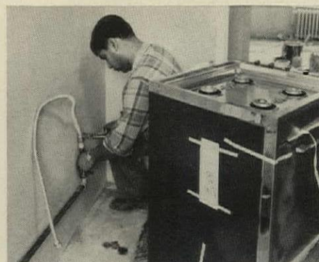
7. RANGE HOOK-UP is completed during first day of remodeling. Tenant thus suffers no interruption in kitchen operation except for water supply, which is still available in bathroom.
