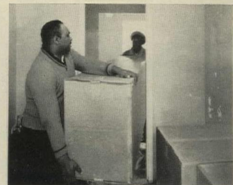
8. NEW EQUIPMENT for second day's work is moved into kitchen on afternoon of first day. Building owner furnishes crew of laborers for this work and removing old kitchen equipment.
