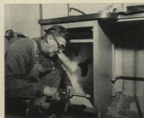
10. PLUMBING HOOK-UP follows cabinet installation. Schedule requires four men for installing cabinets, two men for all other trades. Contract sets holdup penalty of $6 an hour.
