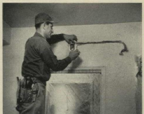
5. NEW OUTLETS are part of updated kitchen design. Electrician starts roughing in as soon as laborers gut old kitchen. Wall clock outlet, shown above, eliminates tenants' extension cords.
