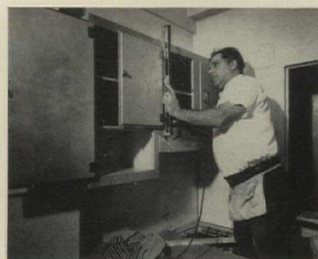
9. CABINET INSTALLATION starts on second day. Work is simplified by stock units with predrilled holes for hardware. To switch lefts or rights, cabinets are turned upside down.
