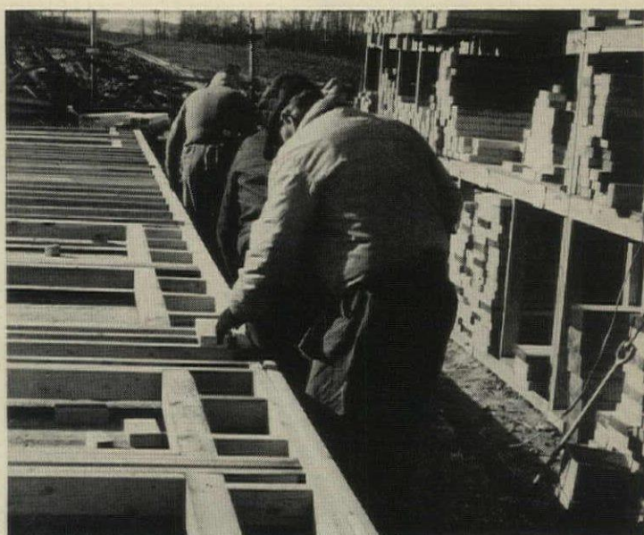
PANELS are assembled on these tables, set 18" high (to accommodate the swing of a man's hammer), then rolled to storage piles.
