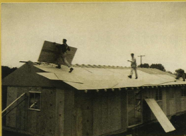
6. As soon as roof sheathing is on, the house is enclosed and doors can be hung. Interior work—which uses as many prefabricated parts and materials as possible—can start any time. It's 1:30.
