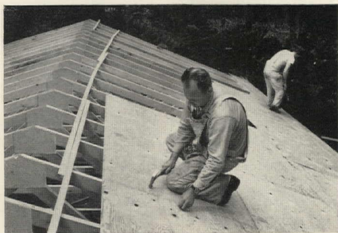
It takes about four man-hours to apply plywood roof sheathing to one of Mitchell's compacts. The house on this page, a little larger than the one at left, has 1,008 sq. ft and sells for about $70 a month on buyer's lot. It's called the "Holly" and was designed by Robert Bruce Waring of the American Plywood Association.
