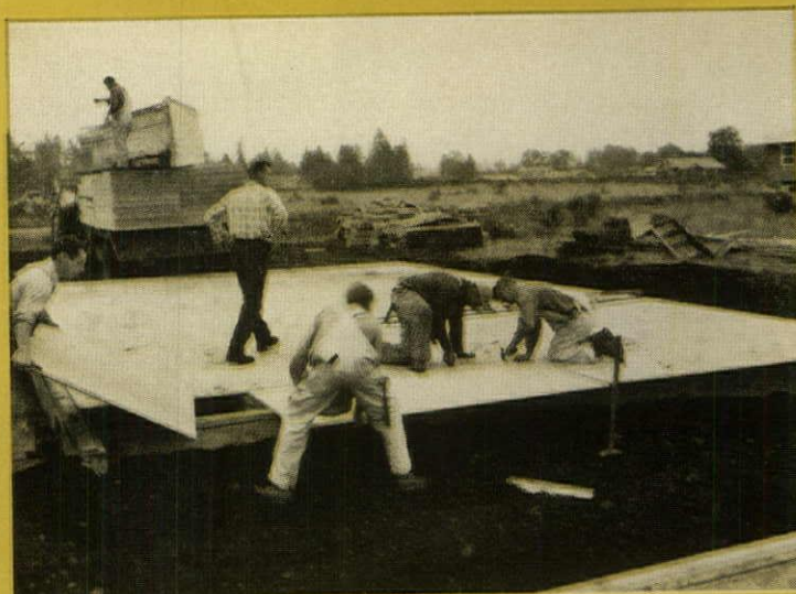
2. The rest of the parts come just as the floor is completed. Buying is simplified because plywood sheathing, wall panels, flooring, trusses and even interior partitions all come from the same supplier.
