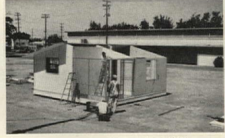
COMPLETED HOUSE costs about $10 per sq. ft. Models range from 500 to 800 sq. ft.
