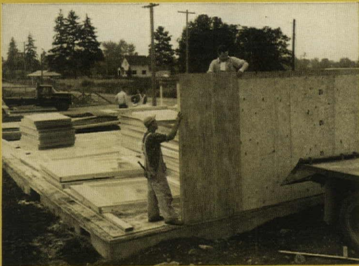
3. Wall components for this M/P model have plywood sheathing on studs; siding will be applied later. Components are stacked on the floor platform near where they'll be used.
