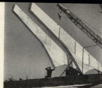
The 44-ft-long plywood box beams, in spite of their strength, are relatively light, 930 lbs. each. It took only two hours to install all seven. They were fabricated by Weldwood Structures Div., United States Plywood Corporation.
