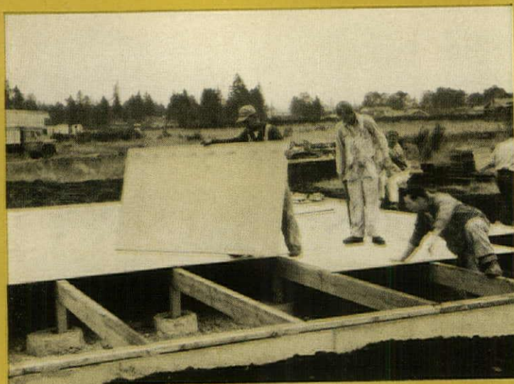
1. Foundation was poured the day before. Plywood floor on this model is 2'4" x 1', the 1 1/8-in.-thick combination subfloor-underlayment, with supports on 4-ft. centers.
