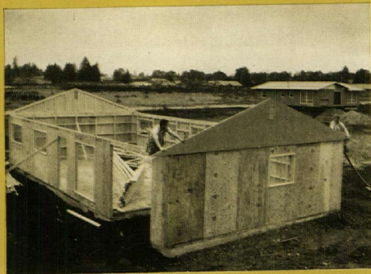
4. By 10:30 (2 1/2 hours after the start of work) the crew is ready to lift prefabricated gable ends into position. Almost at the same time, they begin installing trusses which are waiting inside on the floor.
