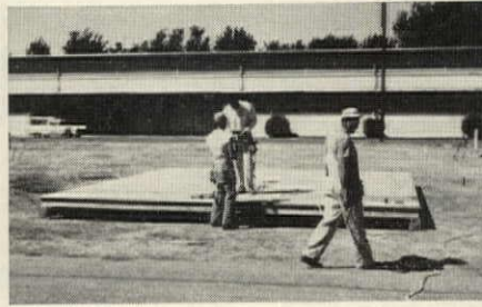
FLOORS are plywood sheets on 2x6s. Panels are 20', the standardized depth of the house.
