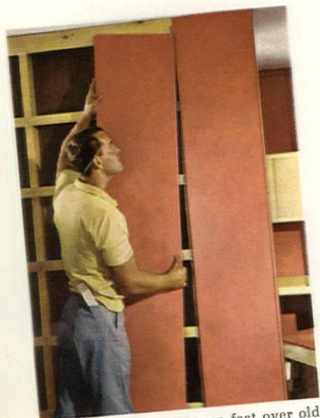
Marlite paneling goes up fast over old walls with little muss and fuss.
