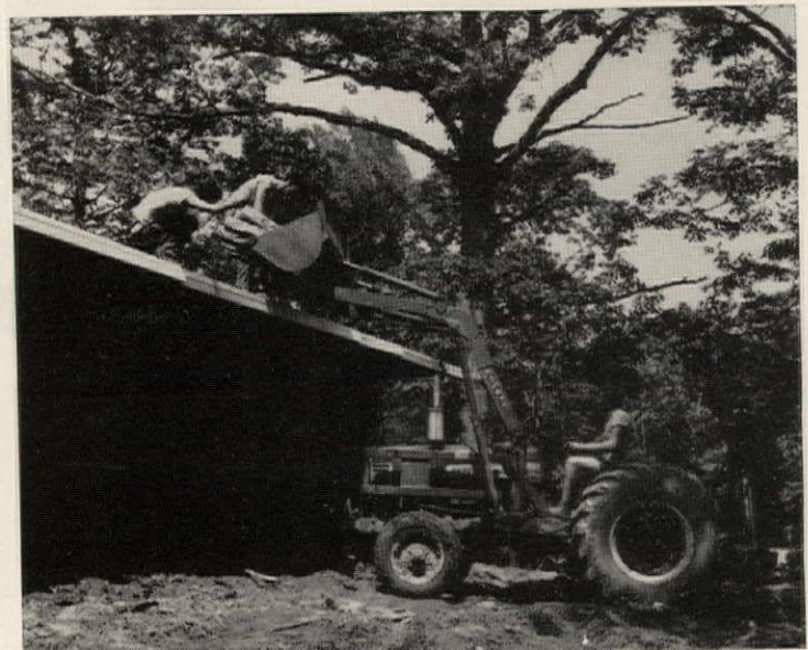
TRACTOR plays a dual role in one of Brosius' subdivisions. Backhoe operator trenching for sewer lateral ( top photo ) stops, places a load of shingles on the roof of an adjacent house ( bottom photo ) and is back on the trenching job within a matter of minutes.
