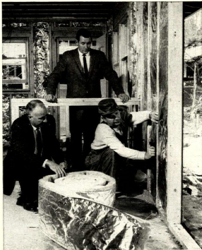
PROPER INSULATION builds in economy and comfort. Here Hobart Smith and construction manager Rousseau check on the installation of full-thick batts in outside walls.
