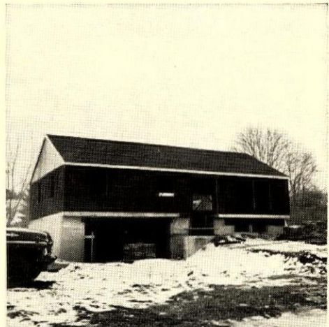
CLOSED-IN SHELL is the result of one day's work by the five-man crew whose schedule is shown at left. Floor deck was already completed when the crew started work. Roof shingles, piled in the garage area, will be applied next day.
