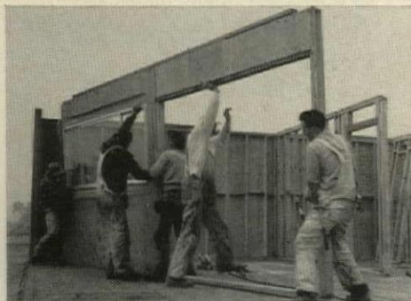
SIX-MAN CREW sets all walls, ready for trusses, at a rate of 1,000 sq. ft. of floor area per hour.
