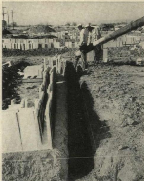
FOOTING IS POURED (see chute, rear) to rough level in trench dug by trencher. Guide lines for top of foundation were staked in after trenching.
