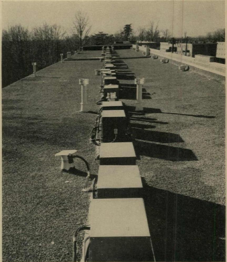
Luxaire Low-Profile Condensing Units hug Southview Apartment roof, serve cooling coils in individual suites through vertical chases.
