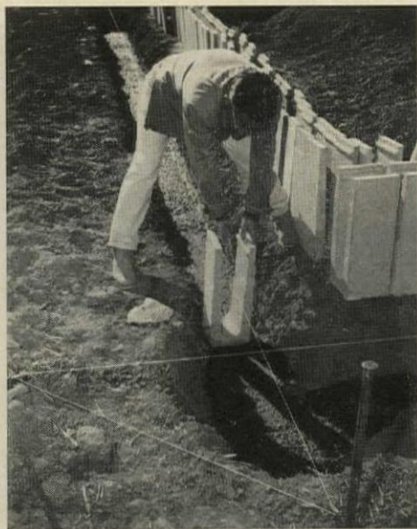
SPECIAL BLOCKS ARE SET into still-wet footing so upper edge aligns with line. Lugs on base of block penetrate into concrete.
