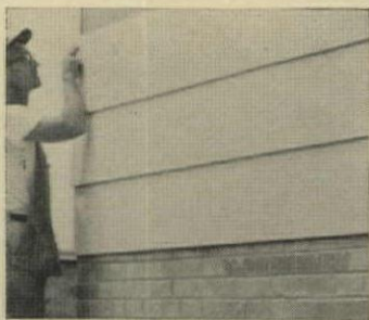
Hardboard siding is primed on all surfaces, has weather-drip edges, and will take any oil-base exterior paint. Horizontal siding is made in 9"x16', 10"x16', and 12"x16' sizes. Wood Conversion Co., St. Paul. For details, check No. 26 on p. 187
