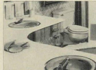
TWIN LAVATORIES can sometimes be run around a corner when there is not enough room for side-by-side installation.
