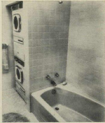
WASHER AND DRYER stacked at end of tub keep down plumbing costs and save the space of a separate laundry.
