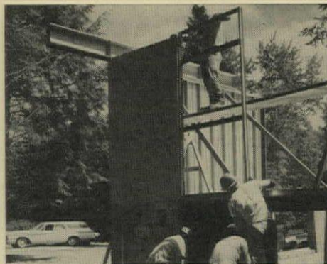
WINDOW FRAME PANEL is bolted to solid panel. Ten-foot cantilevered header, left, is bolted to tops of panels, carries roof overhang.
