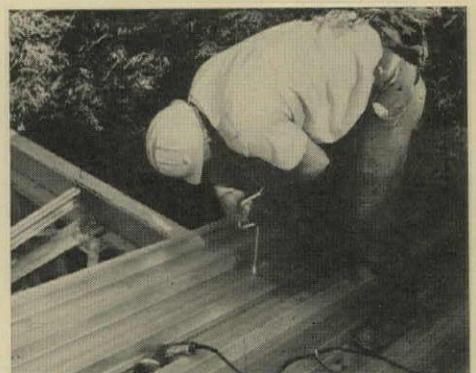
ROOF IS BOLTED to continuous header. Panel is 22-gauge steel with 2-mil aluminum coating on both sides, so no additional finish is needed.
