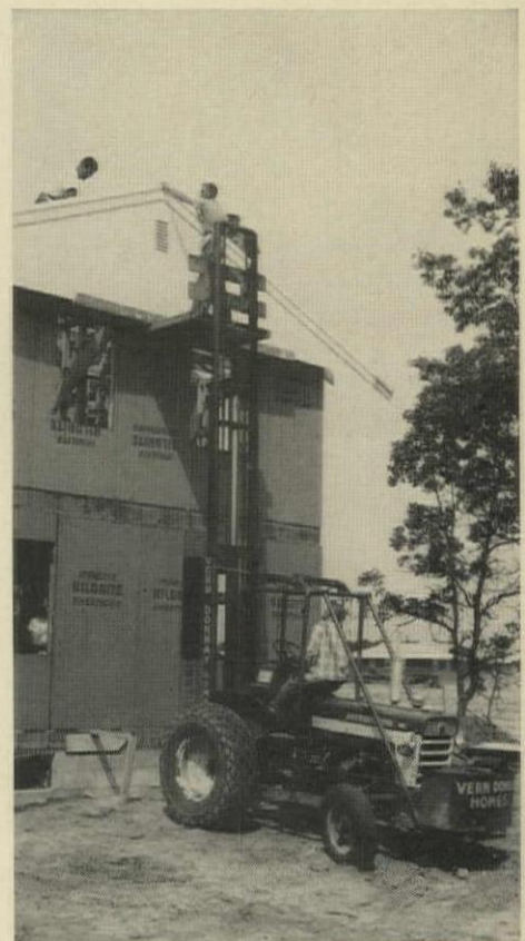
FORKLIFT TRUCK hoists prebuilt gable end to the top of a two-story house, cuts the in-place cost about 25%, says Donnay.
