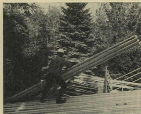
ROOF PANELS are 24" wide, 2" deep, 29' long. Maximum span is 17'. Truss section in center is part of roof-framing system.
