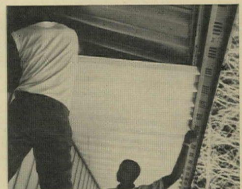
SOFFIT is supported by eave strip, right, and header, left. Section is 16"-wide channel, similar to floor section but lighter.
