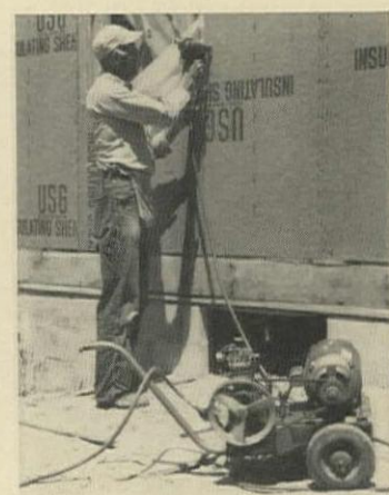
POWER NAILER reduced Donnay’s costs so drastically on sidewall sheathing he ordered two more to nail plywood on decks and roofs.
