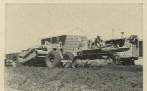
DOZER AND SCRAPER combinations like this allow Donnay to handle all the cut-and-fill operations in his subdivisions.
