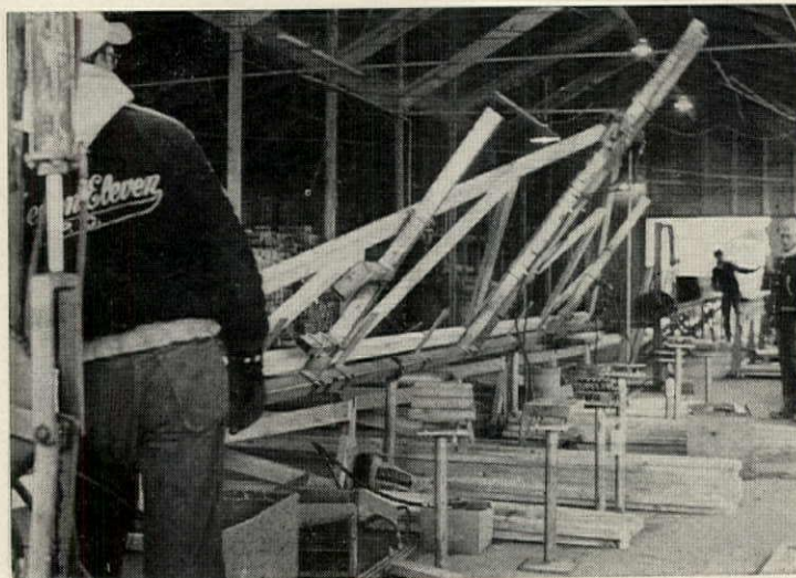
JIG TURNS TRUSS OVER so a second set of metal plates can be tacked to the other side before truss goes through roller press.
