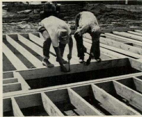
PRECUT JOISTS and prefabbed stair well are nailed into place. Then subfloor is applied.
