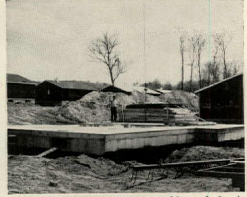
INTERIOR PARTITION LOAD , with roof sheathing on top, is set on corner of deck by crane.
