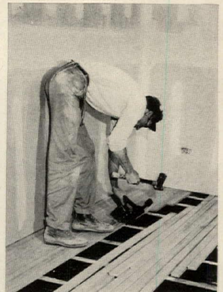
STEP 3. 25/32" strip oak flooring is nailed directly to sleepers formed by double 1 x 2s. Flooring nails go through the bottom 1 x 2s.
