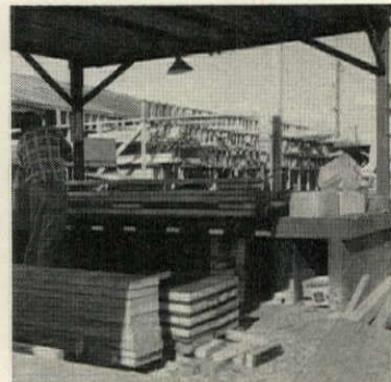
SUB-ASSEMBLY SHOP uses blocking from salvage cutter to make up headers, cripple units, etc, for wall and partition assembly tables.
