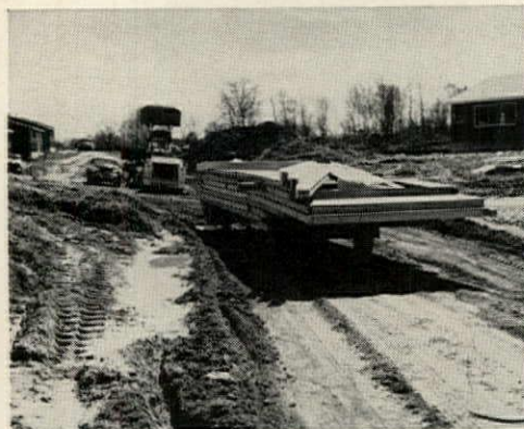
EXTERIOR WALL PACKAGE is stacked so panels needed first are on top.
