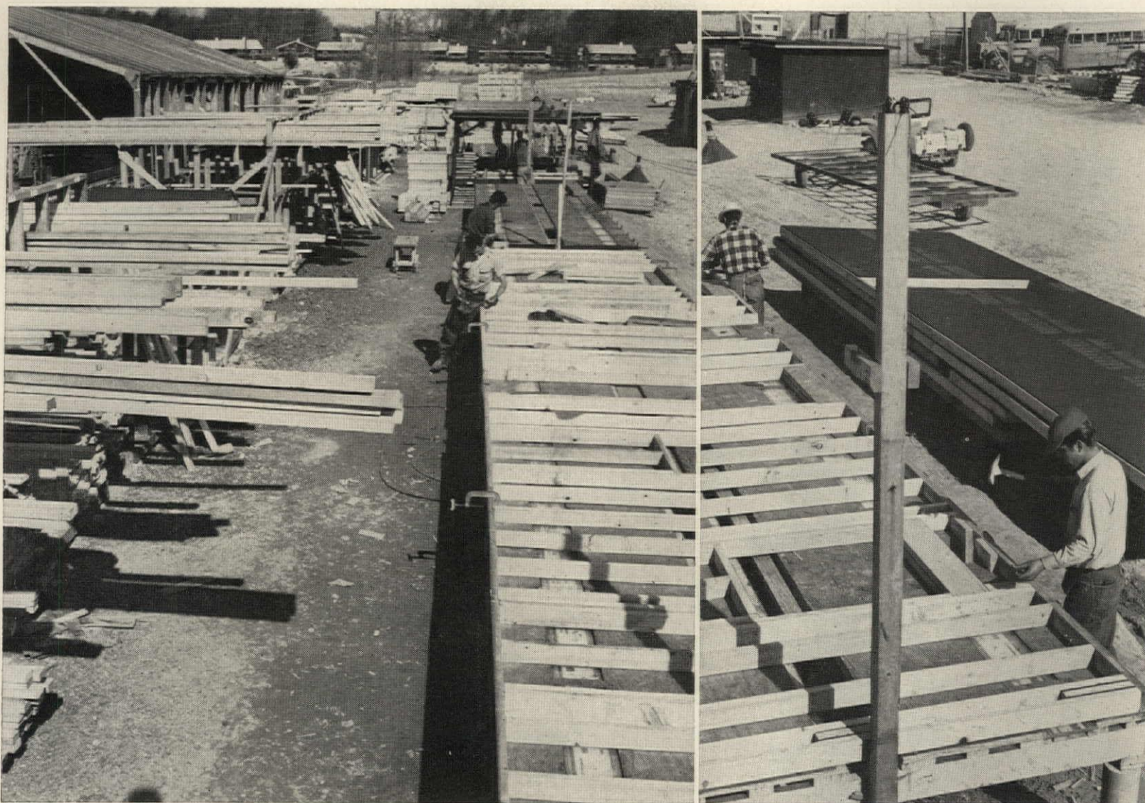
JIG TABLES are used to prefabricate both exterior walls (foreground) and partitions (background). Precut pieces come from storage bins at left; finished components are stacked on trailers, right. Twenty-four
