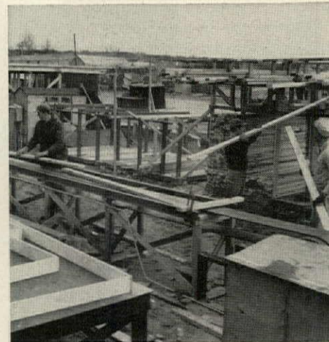
DEFLECTORS , made from scrap lumber, are set up to stop pieces when they reach the proper bin (truss parts are stopped opposite truss jig, etc).
