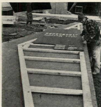
GABLE ENDS are assembled on wooden jig tables just beyond main truss assembly area. Sheathing is nailed with pneumatic hammer.
