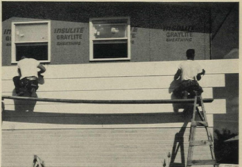
GOES UP FAST. Here's how Medema Bldrs. put it: "Insulite Primed Siding is easy to handle, easy to apply over the rugged Insulite Sheathing we also use. Packages unload from truck quickly—either manually or with fork lift."
