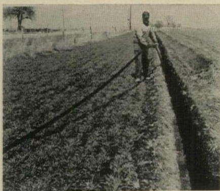
WATER SERVICE LINE is run out in continuous lengths and fed into narrow trench.
