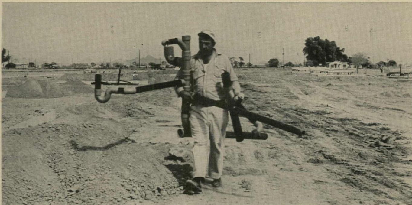
VENT AND WASTE TREE , shop-assembled of ABS plastic off site, is a light load for one man at an Arizona development.
