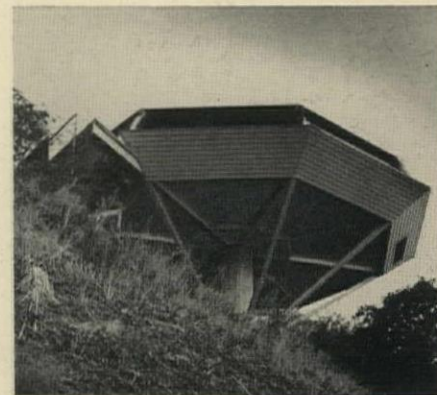
STEEL BRACES tie floor framing to supporting column. House is 60' in diameter.
