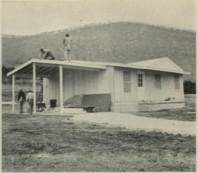
4:30 Houses are erected and closed-in by seven-man crews in 8 hours, and are ready for interior finishing. Prime-coat painting of the exterior components safeguards them from inclement weather.
