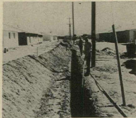
GAS SERVICE LINE is quickly installed in trench along rear lot line of Phoenix houses.
